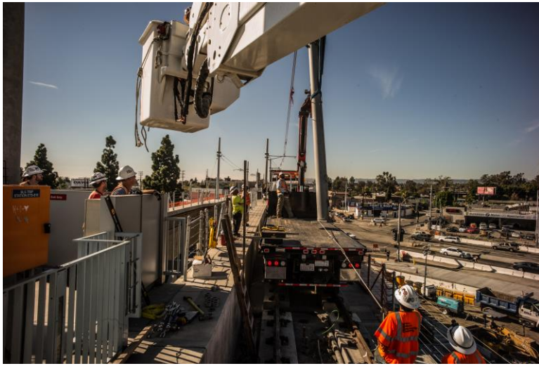
OCS pole removal to make way for Phase 1 and Phase 2 track tie-in
