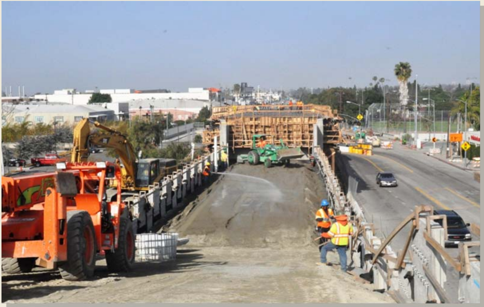
MSE Walls From La Cienega Aerial Structure to Ballona Creek Aerial Structure
