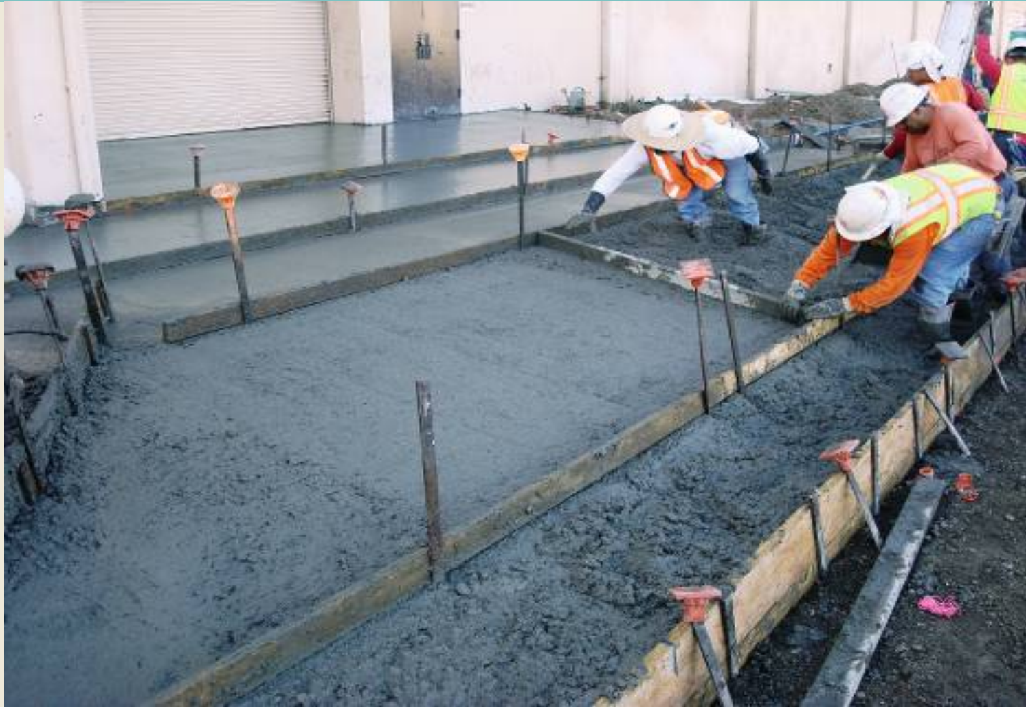
Placement of Concrete for Driveway in Front of LATTC on Flower St
