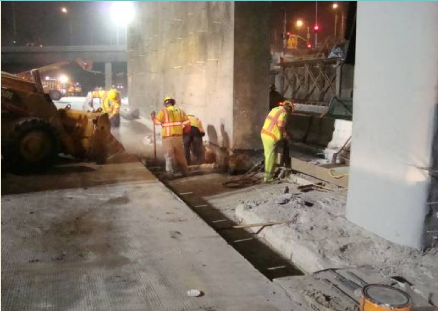
Concrete Replacement at I-110 Freeway Median with Flower St Overcrossing False-Work in Background
