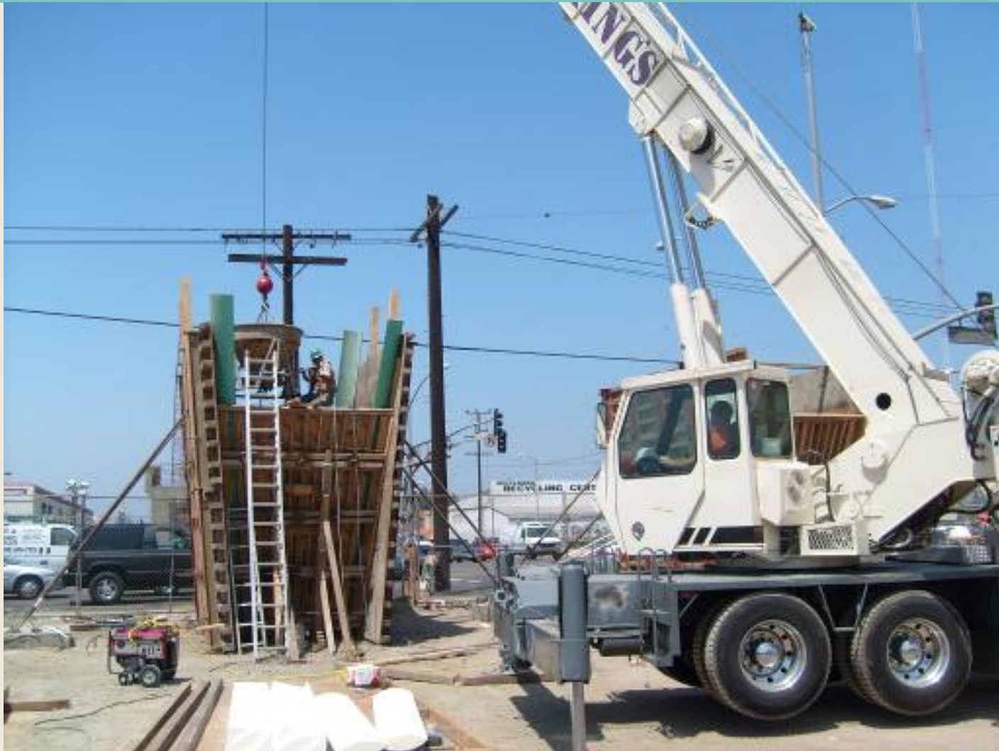
Concrete Placement for Bent No. 4 South Upper Column at La Cienega Overcrossing Structure
