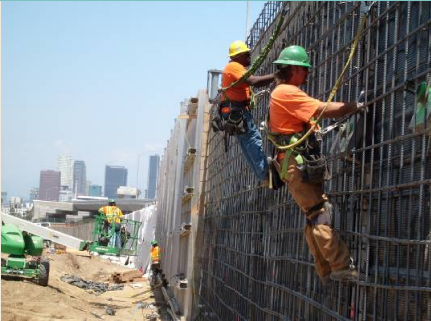
Rebar Installation at Retaining Wall on Flower St North of Jefferson Blvd
