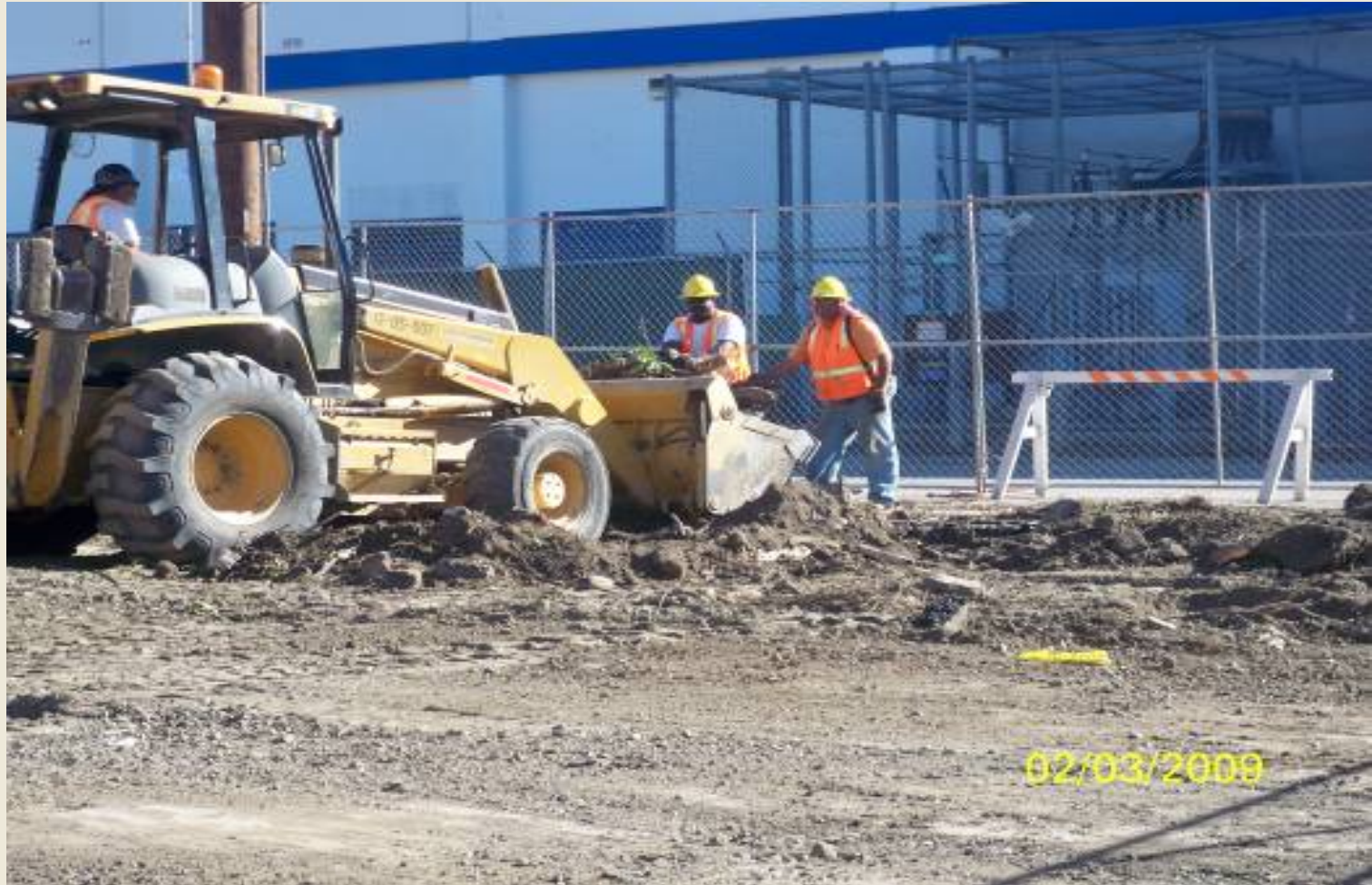
Clearing and Grubbing of Right of Way at La Brea Ave and Rancho Cienega Park
