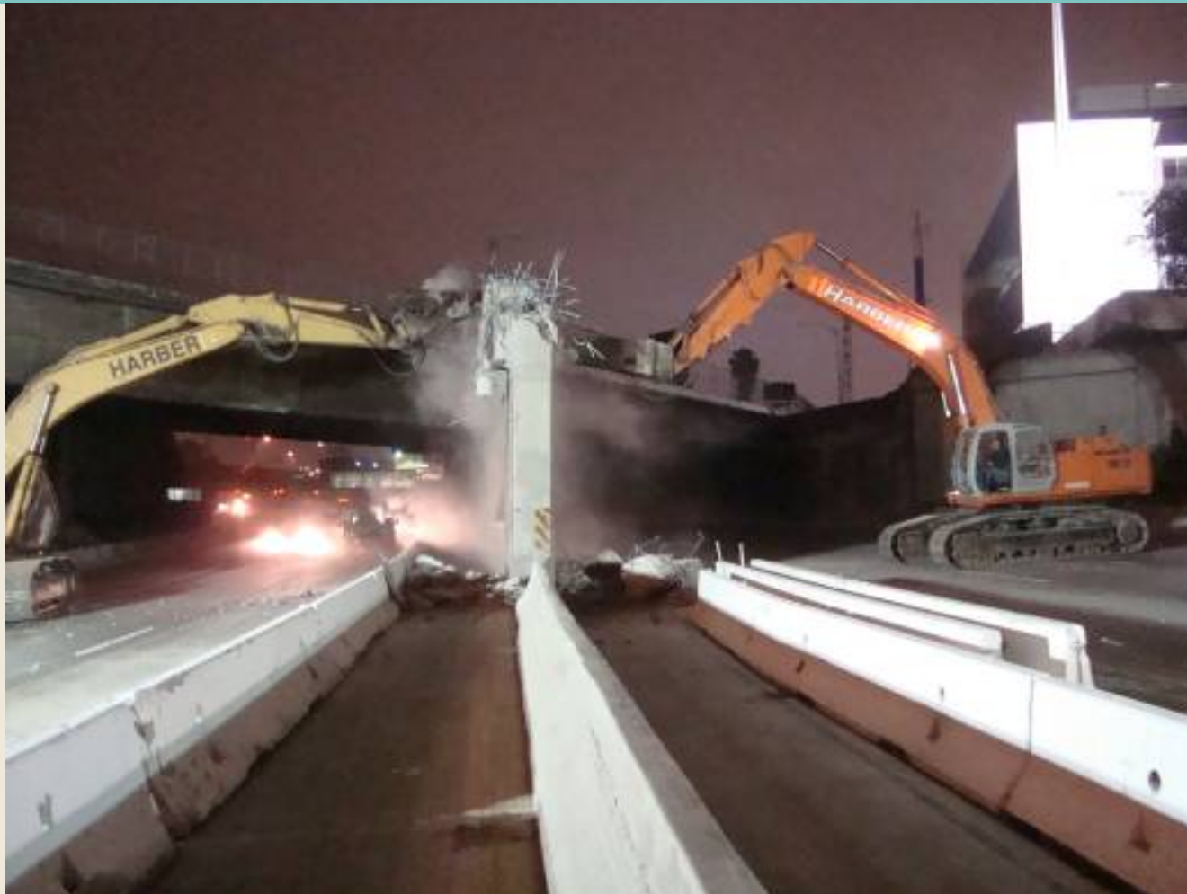
Column Demolition on I-110 Freeway in Preparation for Flower Street Bridge Retrofit
